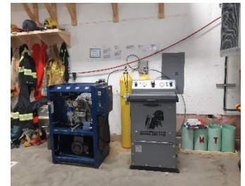
breathing apparatus fill station
